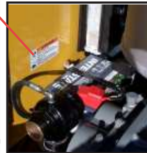
INSIDE DIESEL ENCLOSURE
