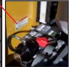
INSIDE DIESEL ENCLOSURE
